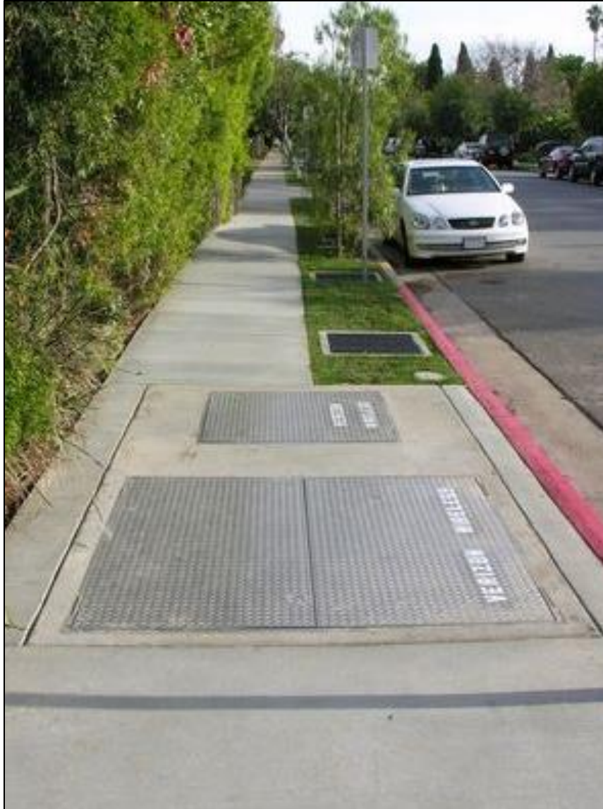
Figure 3: Flush-to-grade underground equipment vault.
