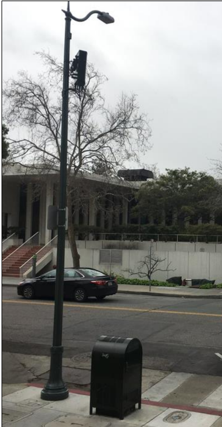
Figure 9: Ground-mounted accessory equipment concealed as a mailbox.
